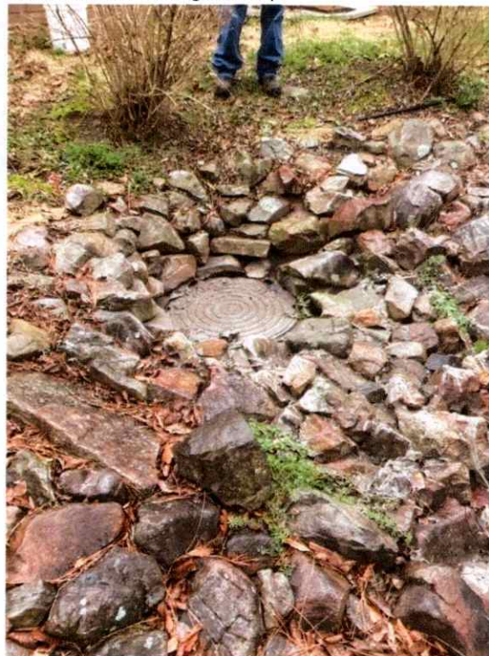
Manhole 3728 – 107 Forest View Court Before Cleanup
