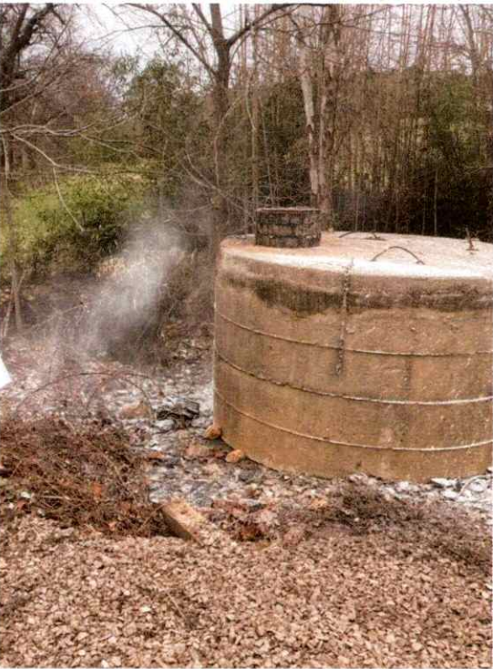
Manhole 1865 - 352 Fontana Road After Cleanup
