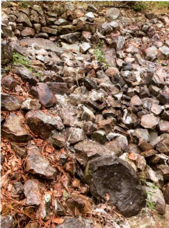
Manhole 3728 – 107 Forest View Court Before Cleanup
